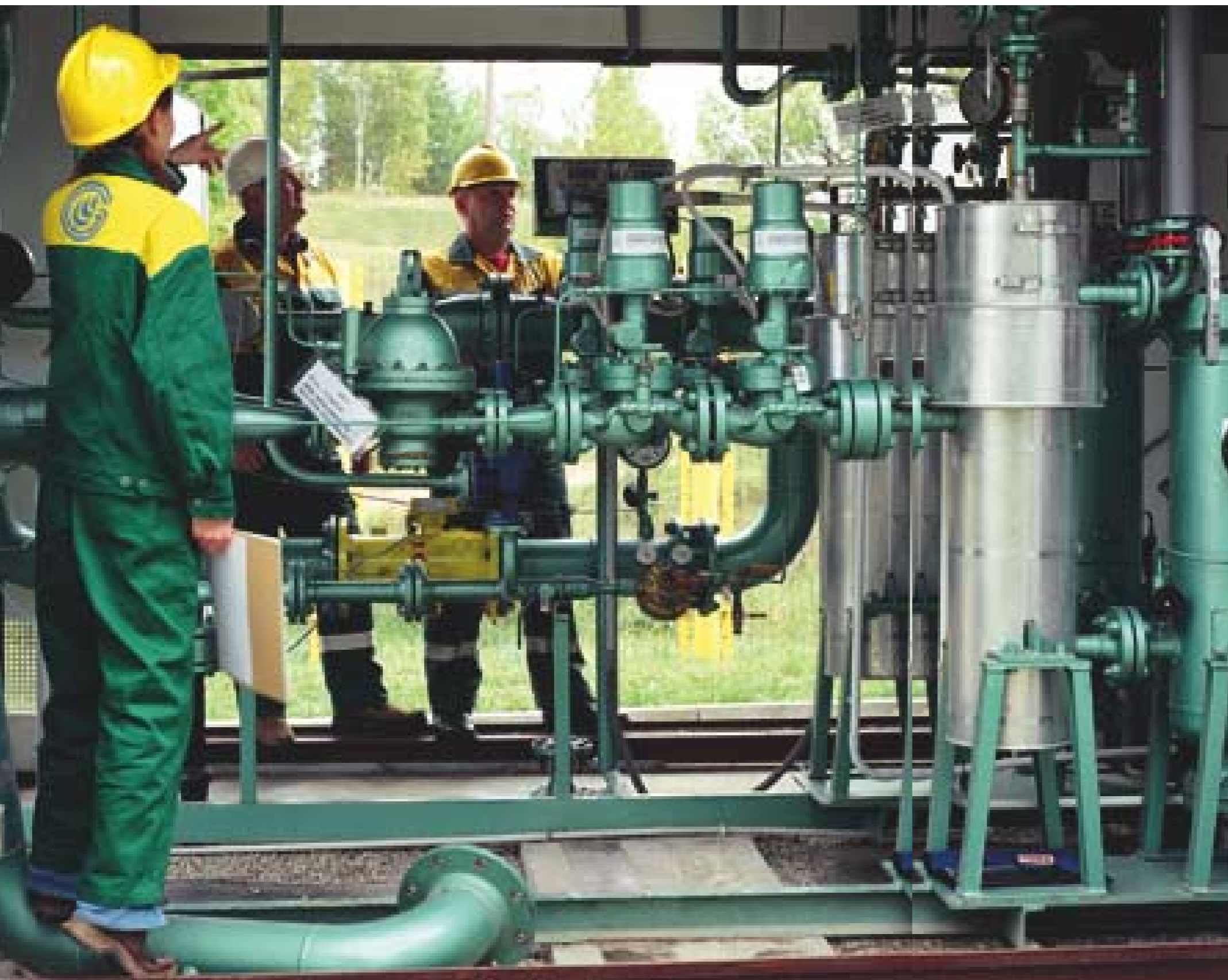
In 2003, the major share of funds allocated for repairs of pipelines and related equipment (65%) was used for the repair of transmission pipelines, their equipment and M/R stations.
