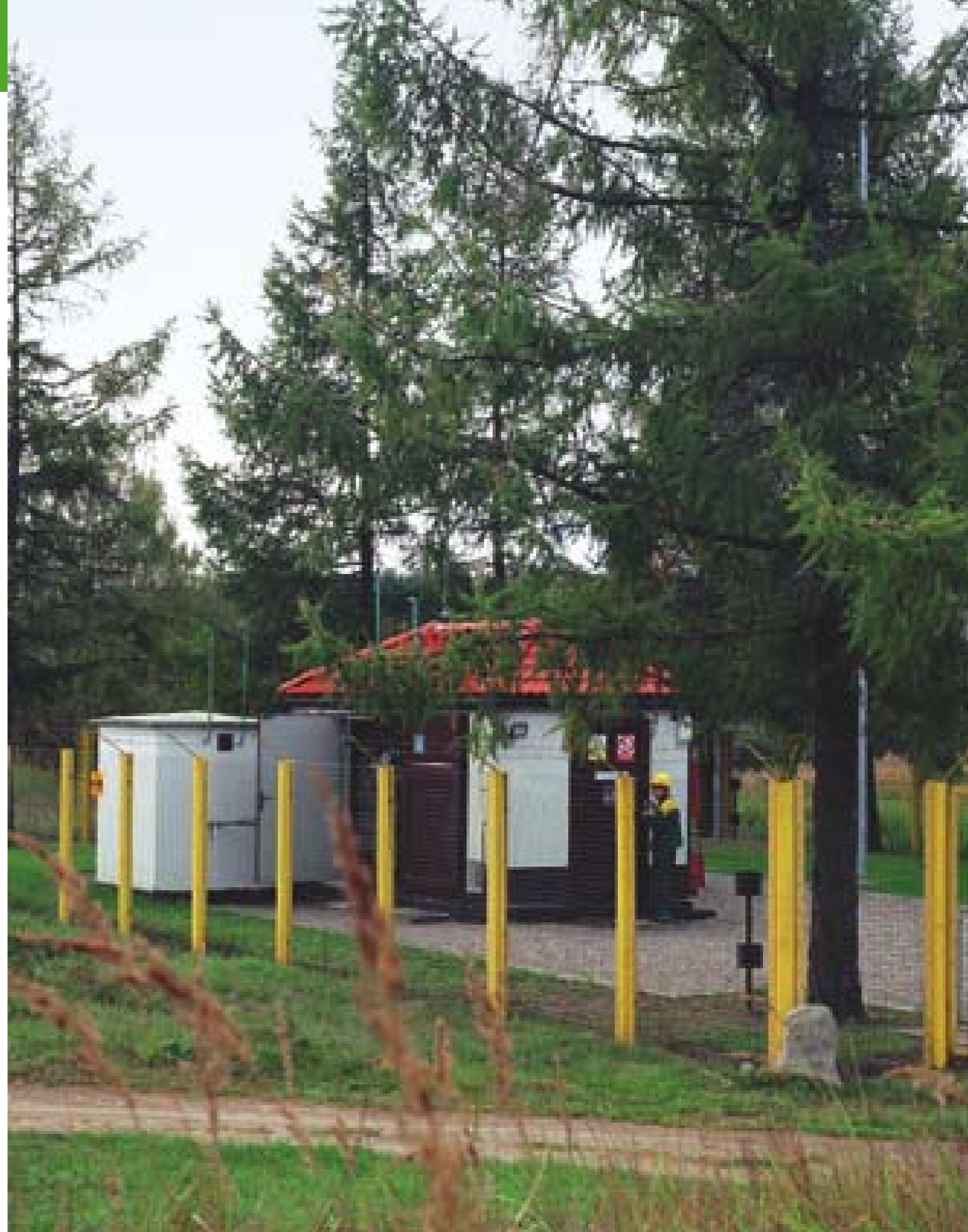
At the end of 2003, all 58 M/R stations of Lietuvos Dujos were integrated into the technological control and data collection system SCADA.
