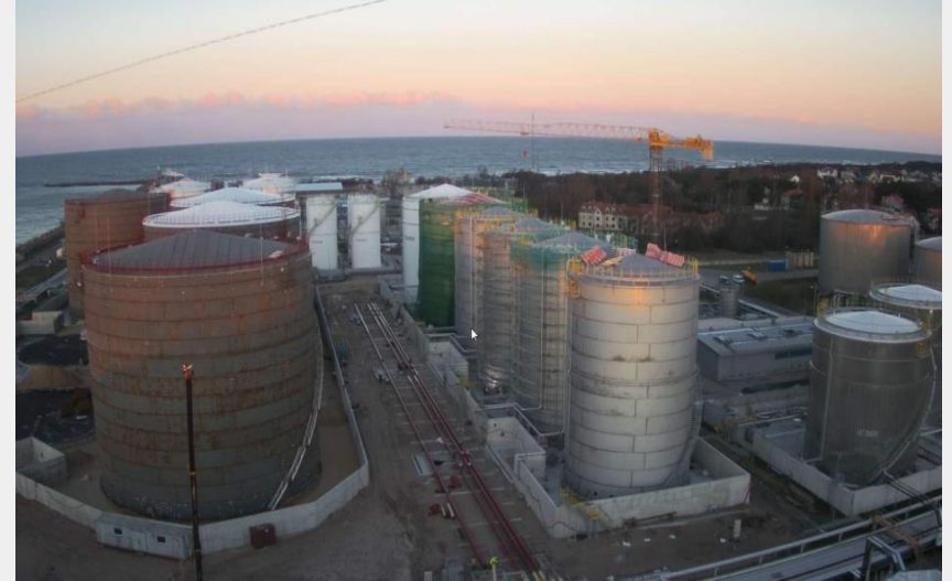
LFO 2 x 10 000 m 3 and 4 x 5 000 m 3 tanks installation - Installation of tanks wall plates and tank park concrete walls ongoing. 2x10 000m 3 tanks erected in full height. Hydrotesting completed. Ongoing with internal painting.
