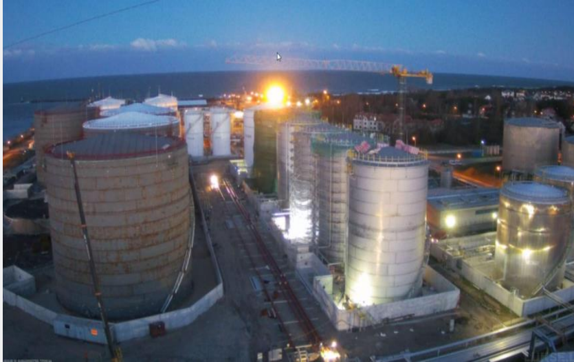
LFO 6 x 20 000 m 3 tanks installation - Installation of tanks wall plates and tank park concrete walls ongoing. Roofs of two tanks painted.
