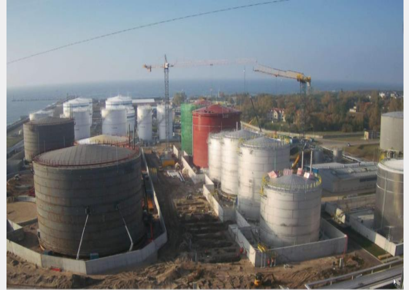
LFO 2 x 10 000 m 3 and 4 x 5 000 m 3 tanks installation - Installation of tanks wall plates and tank park concrete walls ongoing. 2x10 000m 3 tanks erected in full height. Hydrotesting completed. Ongoing with internal painting.
