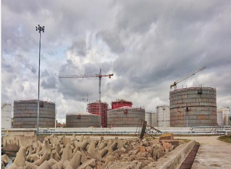
LFO 6 x 20 000 m 3 tanks installation - Installation of tanks wall plates and tank park concrete walls ongoing. Roofs of two tanks painted.
