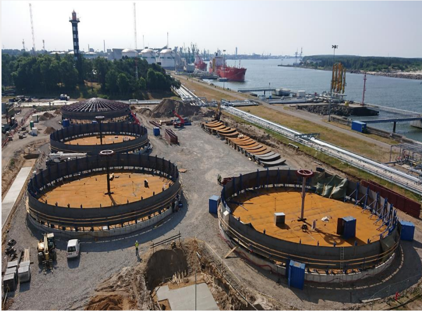
LFO 6 x 20 000 m3 tanks installation - earth works and foundations installation works have been done for 4 out of 6 tanks.
