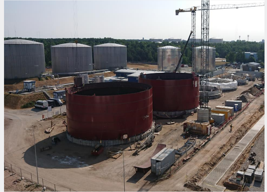
LFO 2 x 10 000 m3 and 4 x 5 000 m3 tanks installation - Earth works and foundations installation works have been done for all tanks.
